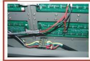
Power line connection inside cabinet
